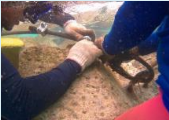
Pamalican Resorts, Inc. Underwater Installation of Cable wire for the Securing of X- Blocks at Cuyo, Palawan
