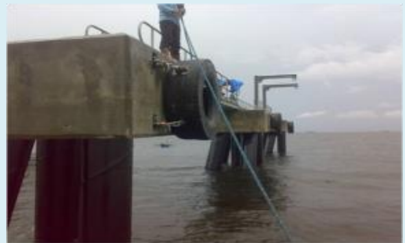
Front side view of the completed Breasting Dolphin Facility at Oilink Int'l., Bataan
