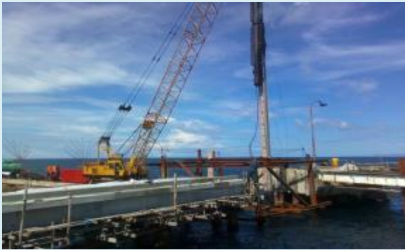
Pile driving activity at the Orca Nitrates Phils, Inc. Pier, Negros Oriental
