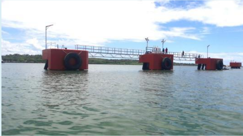
PHOENIX PETROLEUM PHILIPPINES INCORPORATED Panoramic View of Berthing Facility Construction of 6000DWT Berthing Facility
