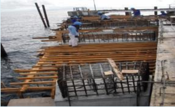
Form preparation for beams of pile caps at the Orca Nitrates Phils, Inc. Pier, Negros Oriental
