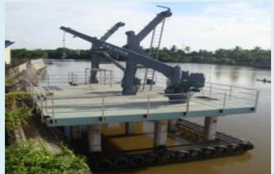
CONSOLIDATED TRAINING SYSTEM, INC. Completed Construction of Mini Pier at Tanza, Cavite
