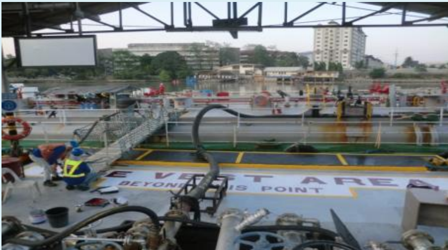
PDSI - Petron Corporation Berthing of Vessel after the Fender Pier Repair at Pandacan, Manila
