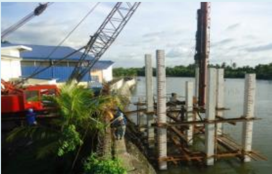
CONSOLIDATED TRAINING SYSTEM, INC. Pile Driving Works for the Construction of Mini Pier at Tanza, Cavite
