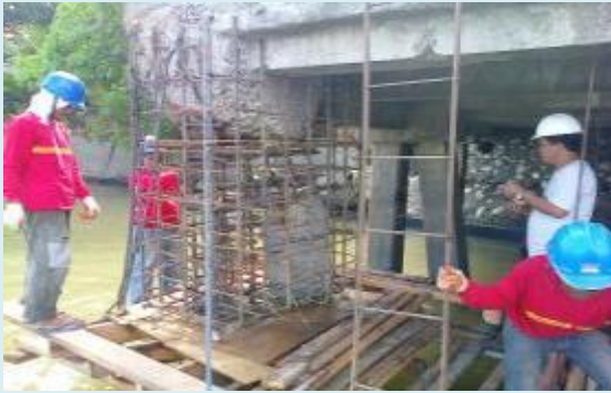
SAN MIGUEL CORPORATION Rebar Installation for the Rehabilitation of Fendering System at SMC Butuan Wharf
