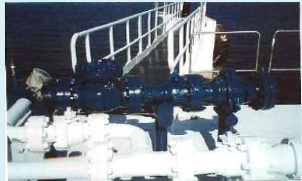
Valve Manifolds at Receiving Platform of 6" \varnothing pipeline and 3" \varnothing pipeline
