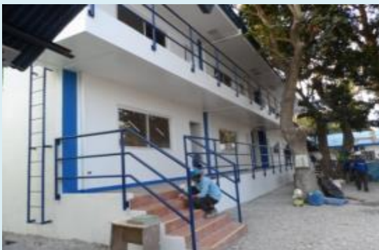
CONSOLIDATED TRAINING SYSTEM, INC. Painting Works for the Construction of Two (2) Storey Classroom at Tanza, Cavite
