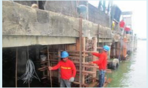
SAN MIGUEL CORPORATION Formworks Installation for the Rehabilitation of Fendering System at SMC Butuan Wharf
