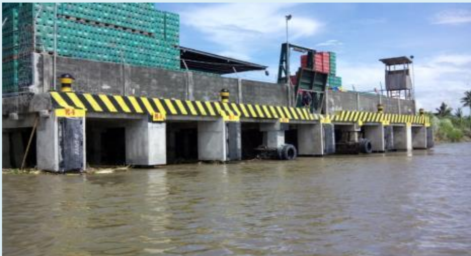
SAN MIGUEL CORPORATION Panoramic View after the completion of Fendering System Rehabilitation at SMC Butuan Wharf
