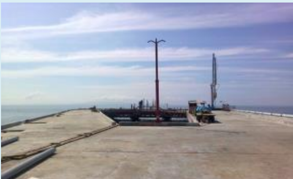
Complete Installation of Fendering System at the Orca Nitrates Pier, Negros Oriental
