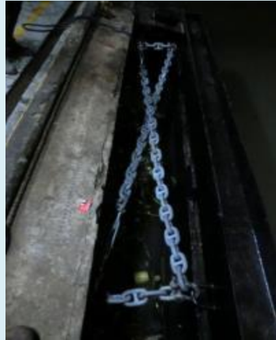
PDSI - Petron Corporation Installation of Chain Link Fender Support at Pandacan, Manila
