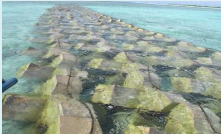
SEVEN SEAS RESORT & LEISURE, INC. Installed Concrete X-Block for Wave Breaker Underwater
