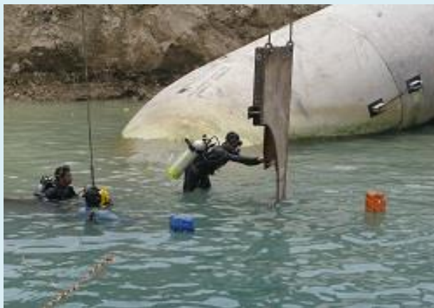
Naphtha Plant Intake Pipe Fitting
